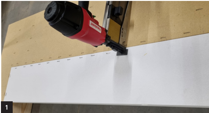
1 Staple COVER PANEL FOR WINDOW LINTELS all round at half the stanchion / waler width
