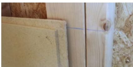
Horizontal alignment of the first row of panels by means of a marking chord.
