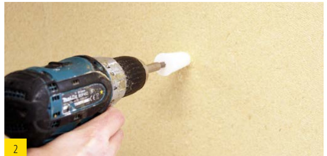
2 Insertion of the spiral anchor by means of a TORX T40 into the unrendered wood fiber insulation board.
