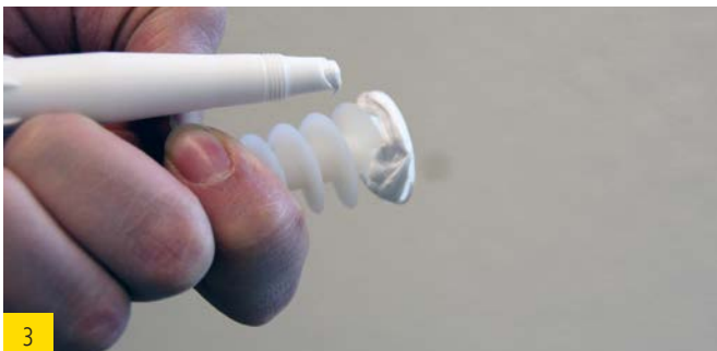
3 Application of best wood FDM WALL gap adhesive sealing compound under the anchor plate.
