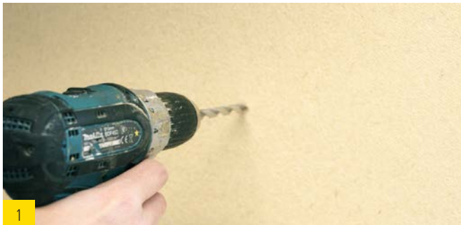
1 Pre-drilling of the unrendered wood fiber insulation board by means of an 8 mm wood drill.
