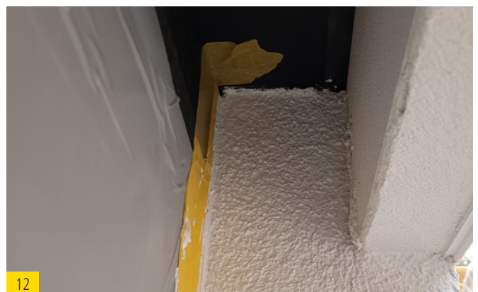
12 The side reveals must be finished with the render system, including paint, up to the top edge of the shaft.
