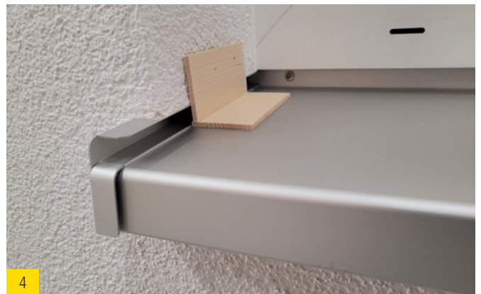
4 Tip: To ensure an even distance to the window sill, use 5 mm shim material (identical to the detailed drawing and order).
